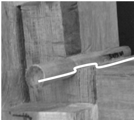
Figure 13 Cross-section of mortise and tenon joint showing small bent and cracks in wood dowel with no obvious crack in the tenon
